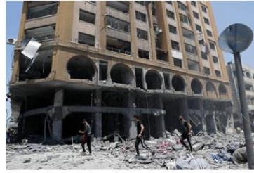
People inspect the rubble of a damaged building which was hit by an Israeli airstrike, in Gaza City, Wednesday, May 12, 2021. (AP Photo/Adel Hana)
